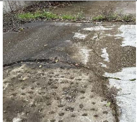
堰体破损、裂缝
