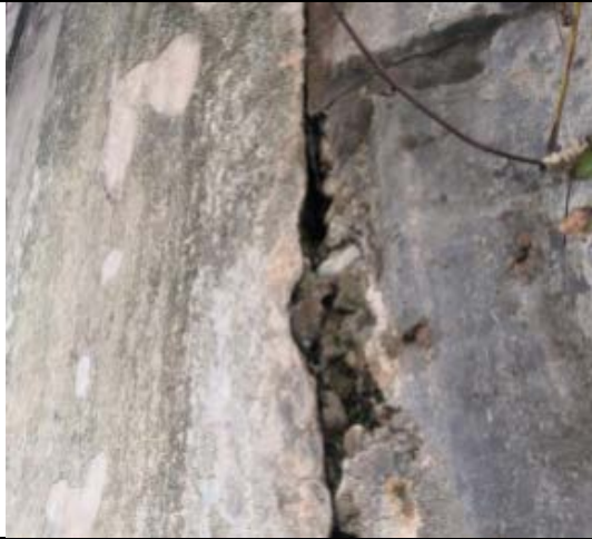
边墙缝止水破坏
